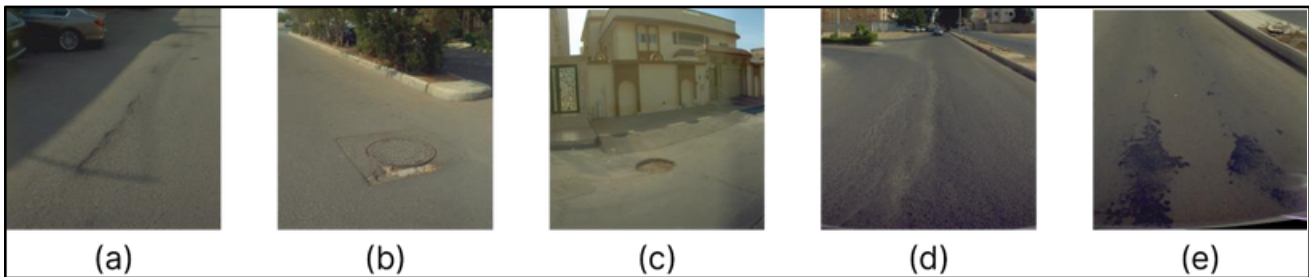
Figure 8: Awes Ebn Thabet road condition; (a) Rutting along with raveling, (b) Poor patch around manhole, (c) Depression in manhole “acts as a pothole”, (d) clear severe weathering and raveling distresse, (e) bleeding.
