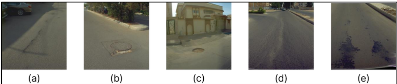
Figure 8: Awes Ebn Thabet road condition; (a) Rutting along with raveling, (b) Poor patch around manhole, (c) Depression in manhole “acts as a pothole”, (d) clear severe weathering and raveling distresse, (e) bleeding.
