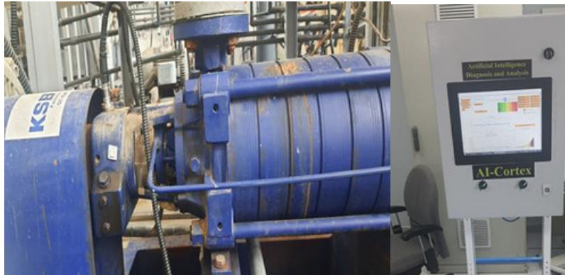
Figure 1. sensor installation on the pump and system installation
