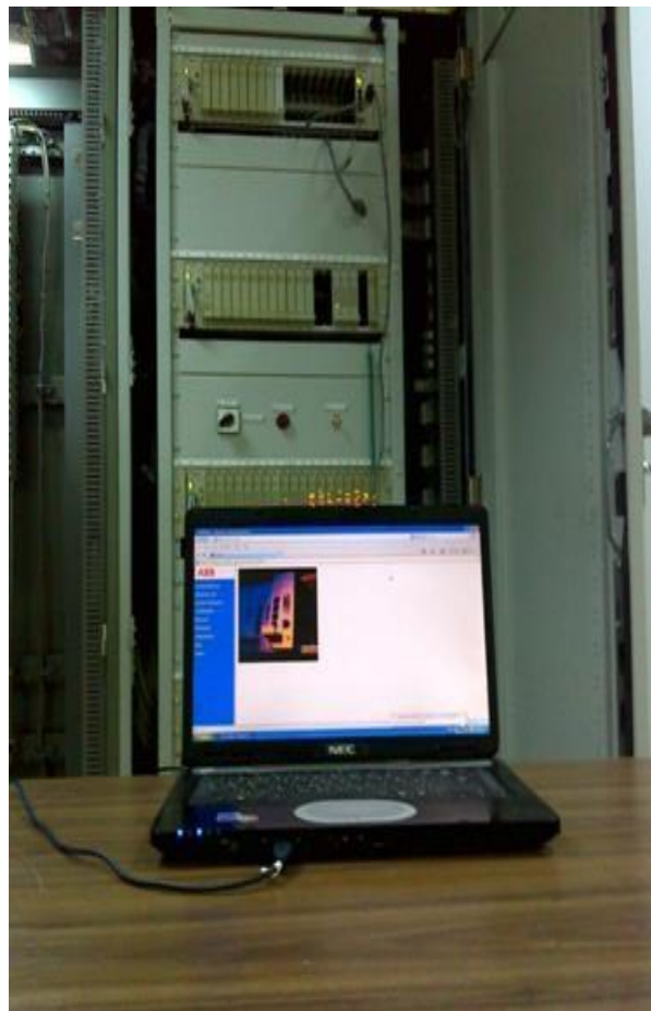
Figure.4: Accessing the RTU locally at Substation with Laptop.
