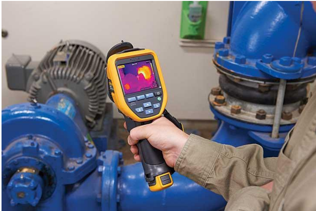
Fig. 3: Thermal imaging as a temperature measurement technique for centrifugal pumps [6].
